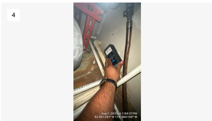
Dry moisture readings indicate singular occurrence or non active leak source.
